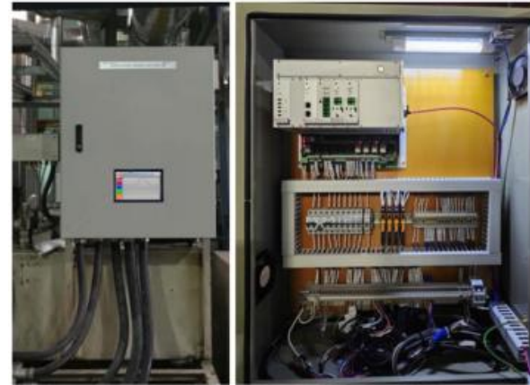
Position Control System
